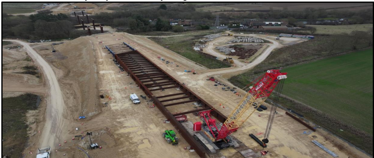
GSRR – Fabrication of the first section of bridge between west abutment and Pier 1
